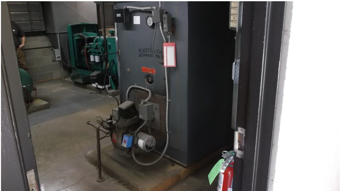
Boiler just inside of door to mechanical room.
