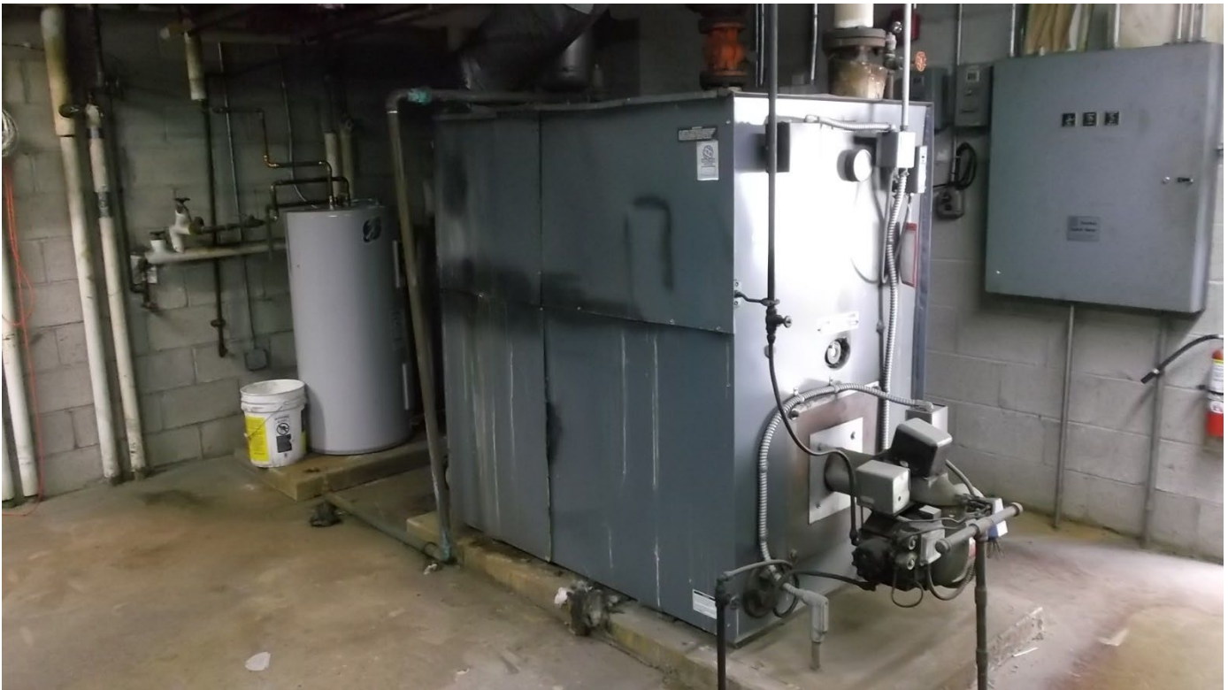
More boiler photos.
