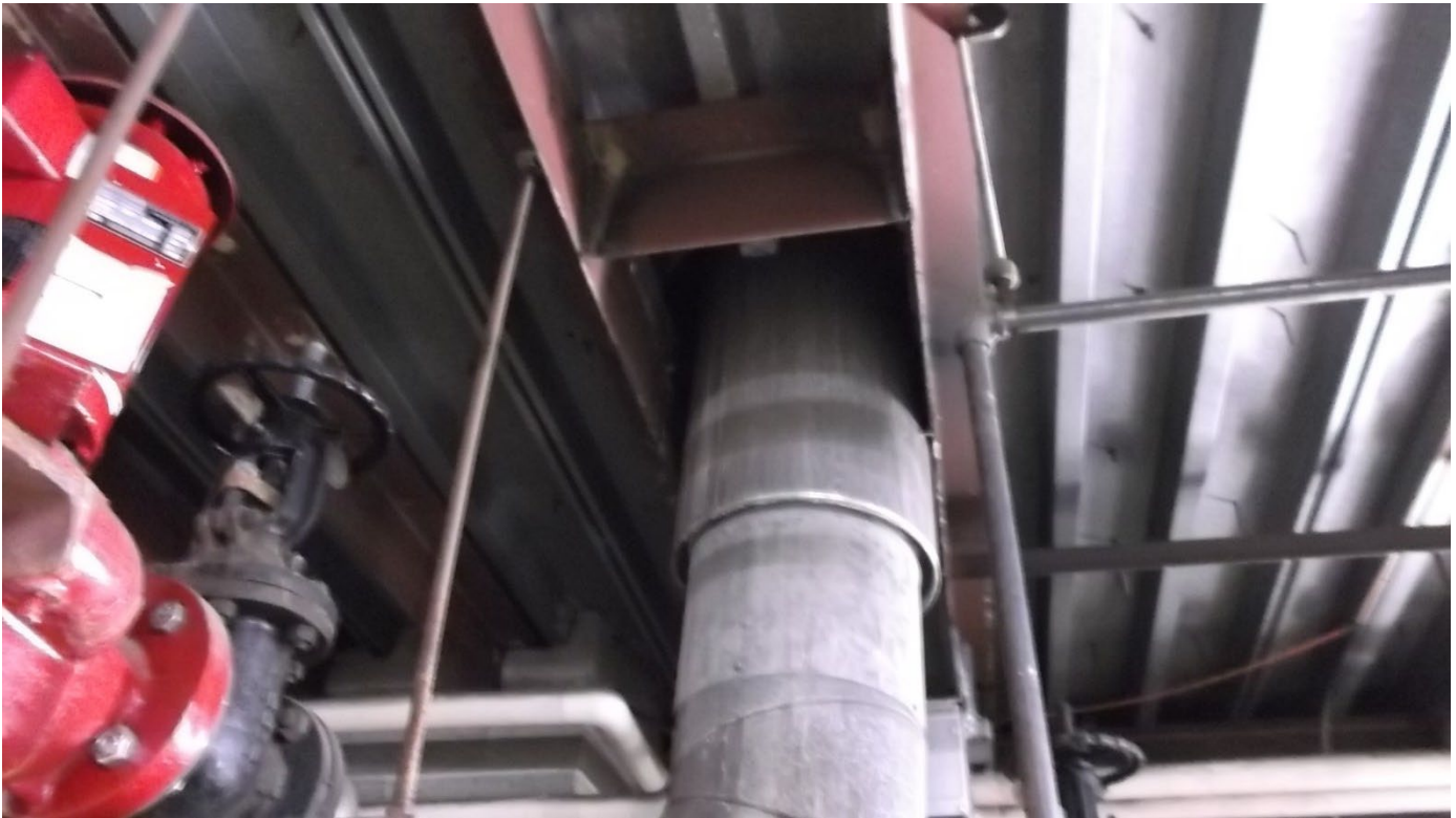
Boiler exhaust stack.
